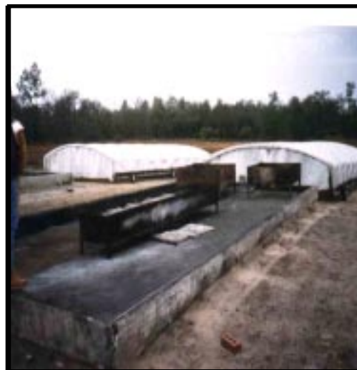
Closeup view of burning pans on concrete slab. Note the white covers in the background which can be rolled over the pans to prevent precipitation from entering them.
