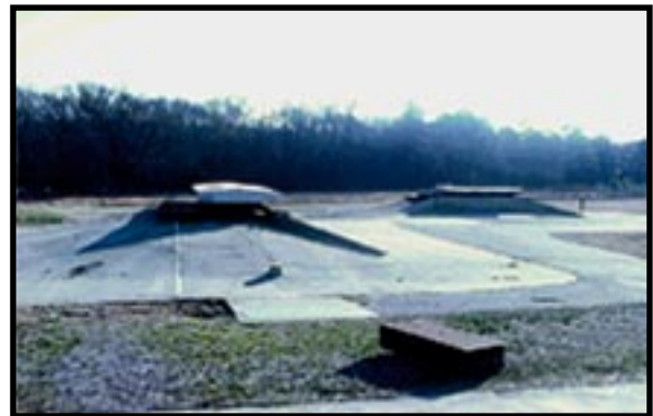
View of burning pans on a secondary containment pad. Note that the pads do not appear to have berms around them.
